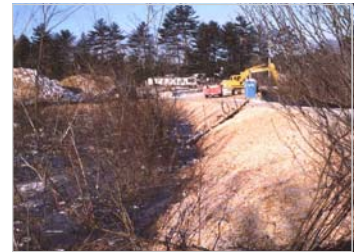
Constructing a wetland for mitigation in Hillsborough. GES designed the wetland as wildlife habitat.
