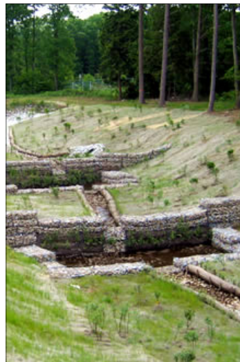
A stream restoration project in Exeter, NH designed by Randall Shuey of the GES Concord office.
